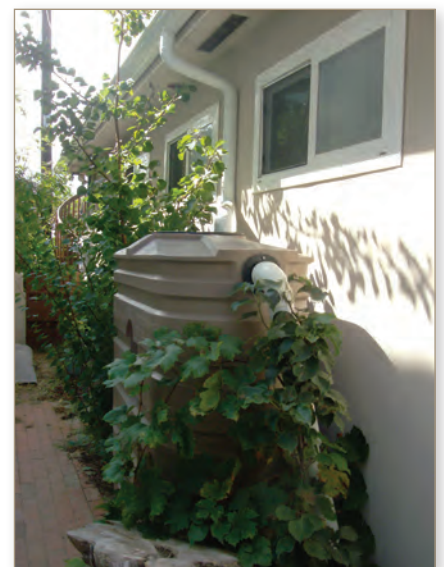
A 300-gallon rain barrel with an overflow pipe that discharges to a landscaped area.
